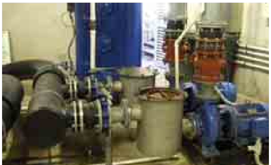
The pump stations have been set up to filter and treat recycled water used on site. The waterfall has its own water supply that is filtered through a Toro 4 Tank Media system then Ozonised and returned to the top of the waterfall.
